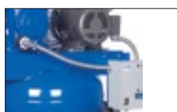
Low oil level switch and magnetic starter
